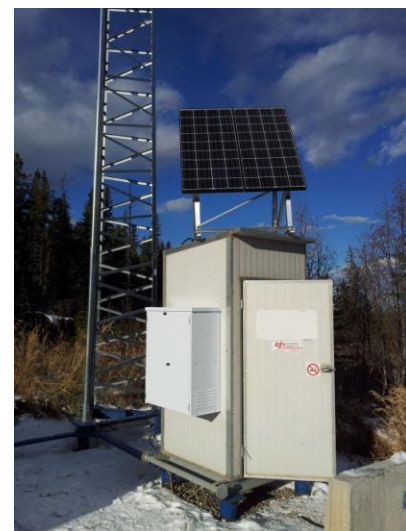
Devon Repeater Site
