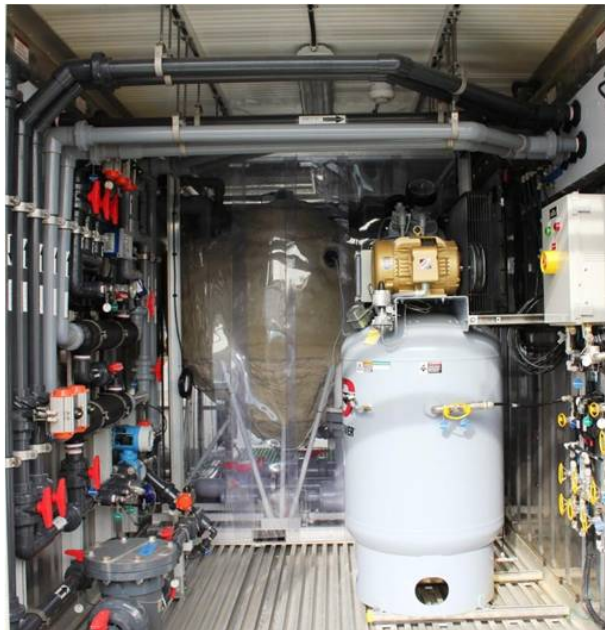
Figure 11: Air Compressor and Heat Recovery
