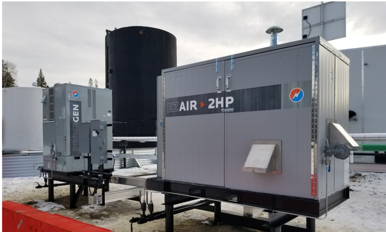
Figure 15 - EZ Air 2hp with M5 installed in Alberta
