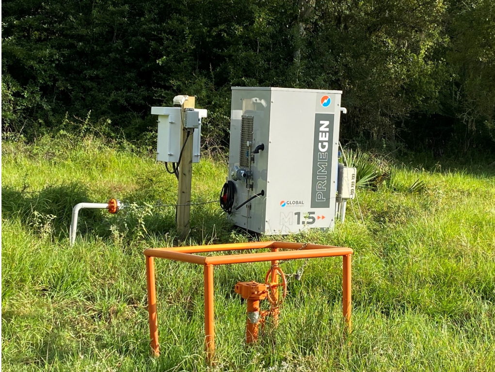
Figure 12 - M1.5 Unit (Texas Site #1)
