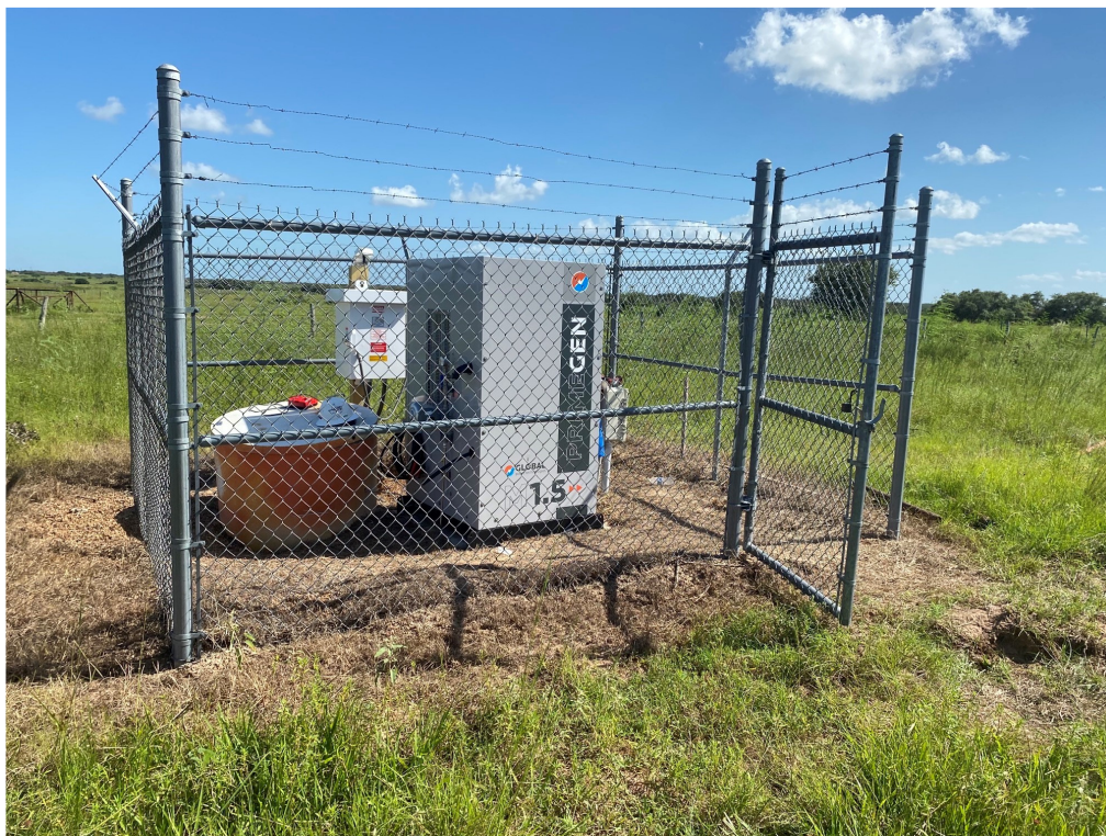
Figure 13 - M1.5 Unit (Texas Site #2)
