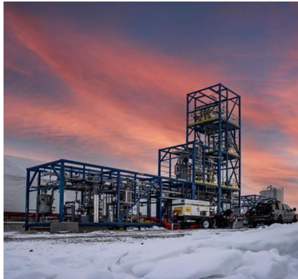
Figure 4: Sunset Photo of Imtex's Commercial Scale 8040 Permylene System
